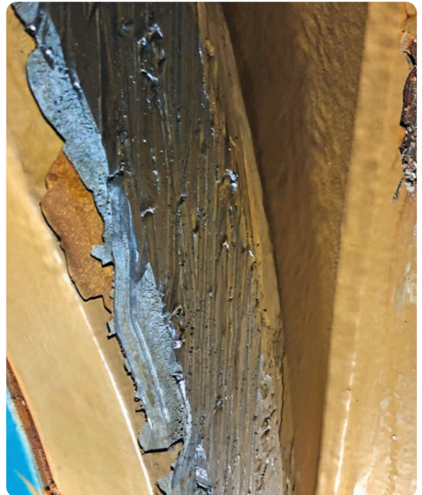
Galled material on valve face
