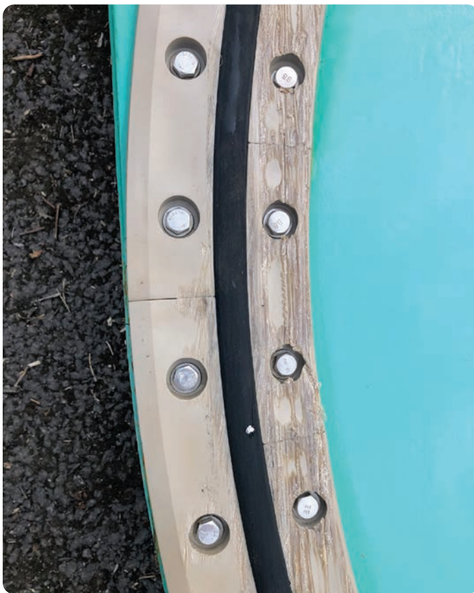
Damaged valve face
