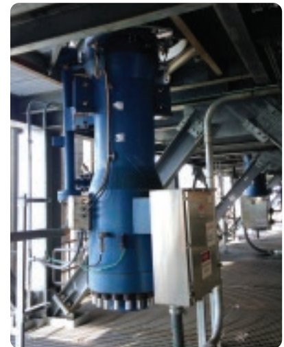
Radiant Syngas Cooling circulating pumps installed in Edwardsport, IN
