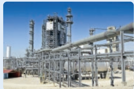
Integrated Gasification Combined Cycle (IGCC) Facility at Edwardsport, Indiana
