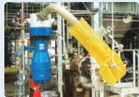
Butanediol reactor recycle pumps installed in LaPorte, TX since 1997
