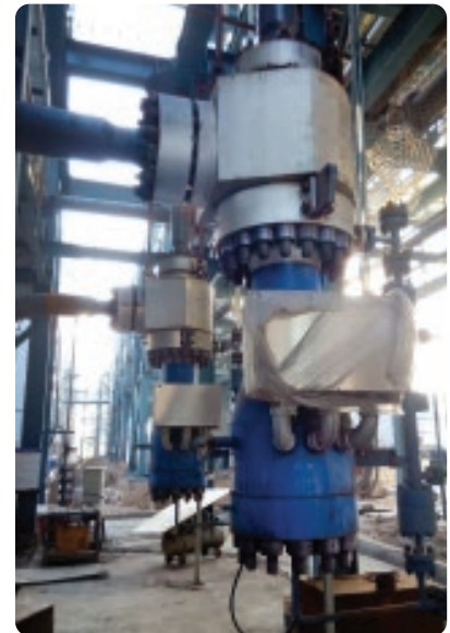
200 HP, 5,800 psi designed BDO reactor recycle pump installations in China
